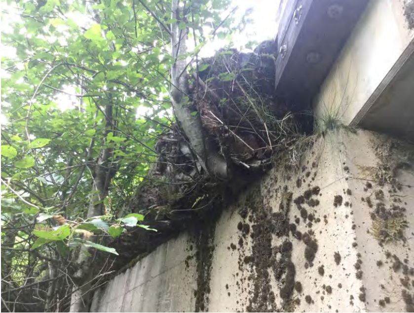
Right Bank Downstream Corner - Rotten Log & Lashing Supporting Fill
