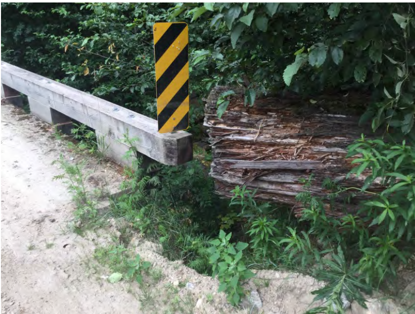
Erosion of Bank Fill at Left Abutment Upstream Corner. Note Rotten Guide Log.
